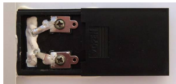
Open Junction Box
